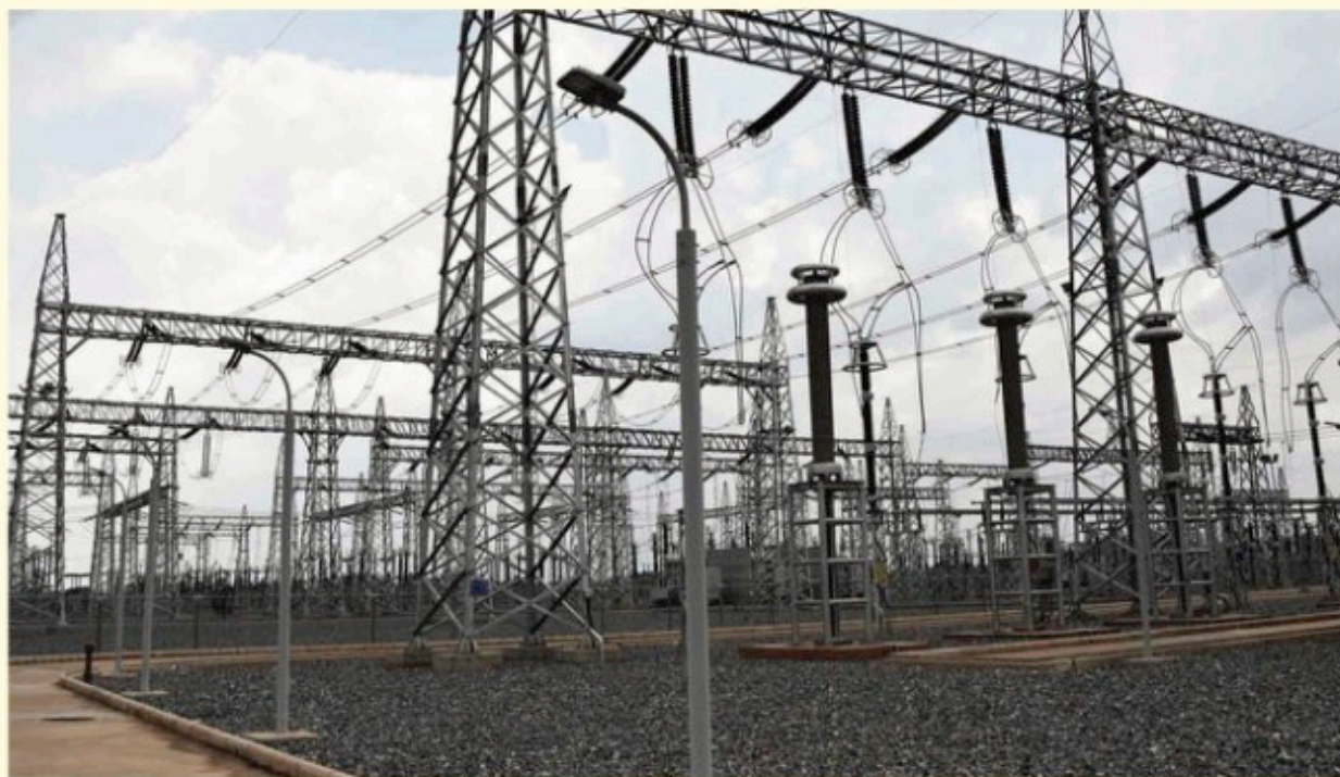
Karuma Hydro transmission lines
